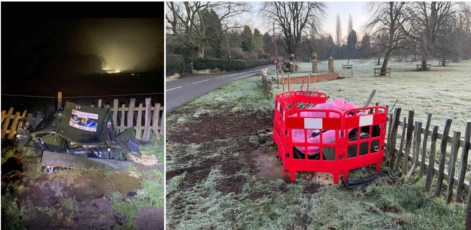
Fig. 18: The Tixall Village BT distribution box (adjacent the village green and obelisk) was demolished twice due to vehicle collisions. This resulted in local residents and businesses losing phone lines and internet connections for weeks. The photo was taken on 12-JAN-2022.
